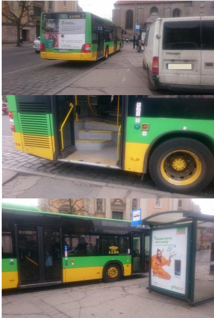
Fig. 7. Stop Bernardyński Square is maladjusted to the needs of the elderly and disabled persons due to: an uneven surface, lack of marking the stop with paint and a warning texture, not adjusted stop height to low-floor buses. Nearby parked cars are additional obstacles on the road (2018). Own elaboration
