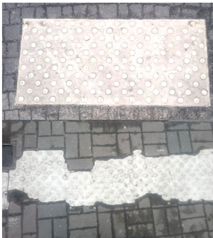
Fig. 12. Examples of warning textures in the public space of Poznań. Lower photo shows worn texture which should be replaced by a new one (2018). Own elaboration
